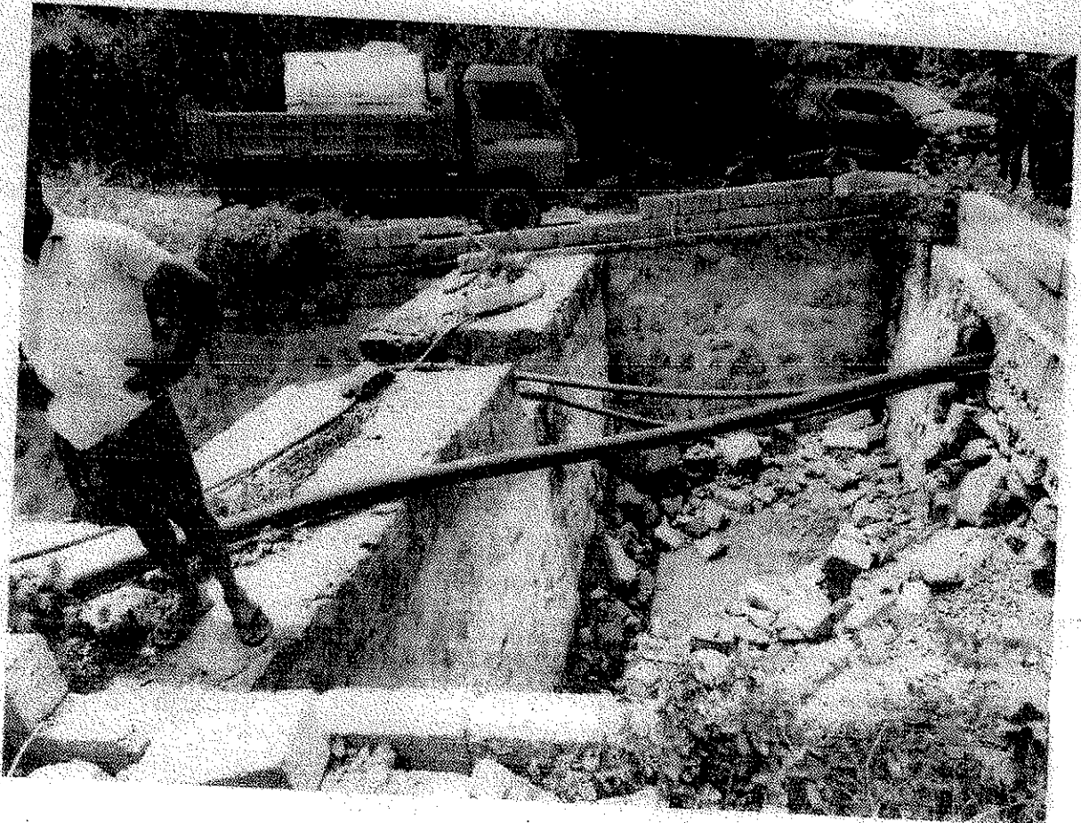
Siltation tanks - Not in use - water from quarry pit bypassed through pipelines to nearby land.
